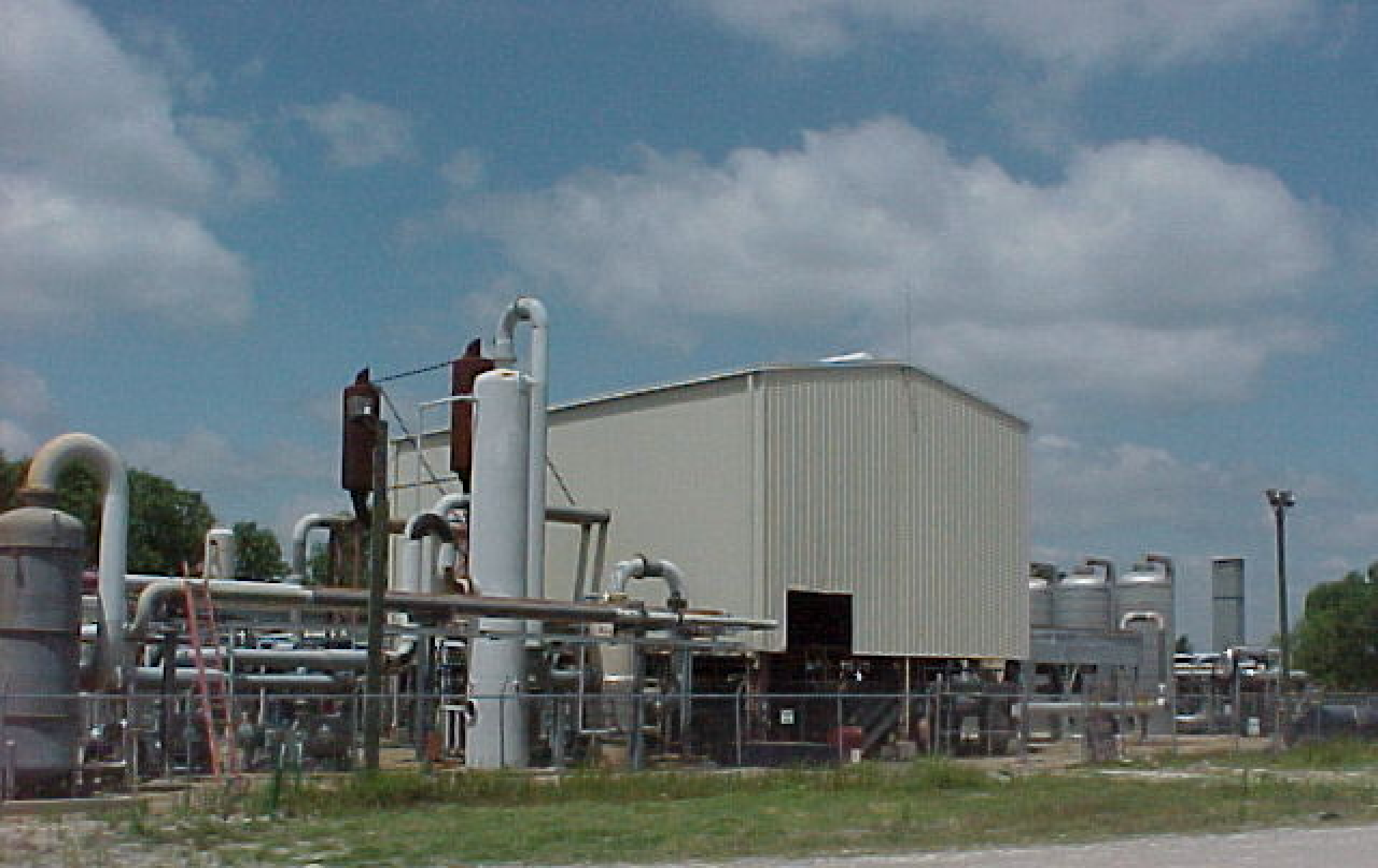
Landfill Gas Processing Plant – on 2-acre tract
