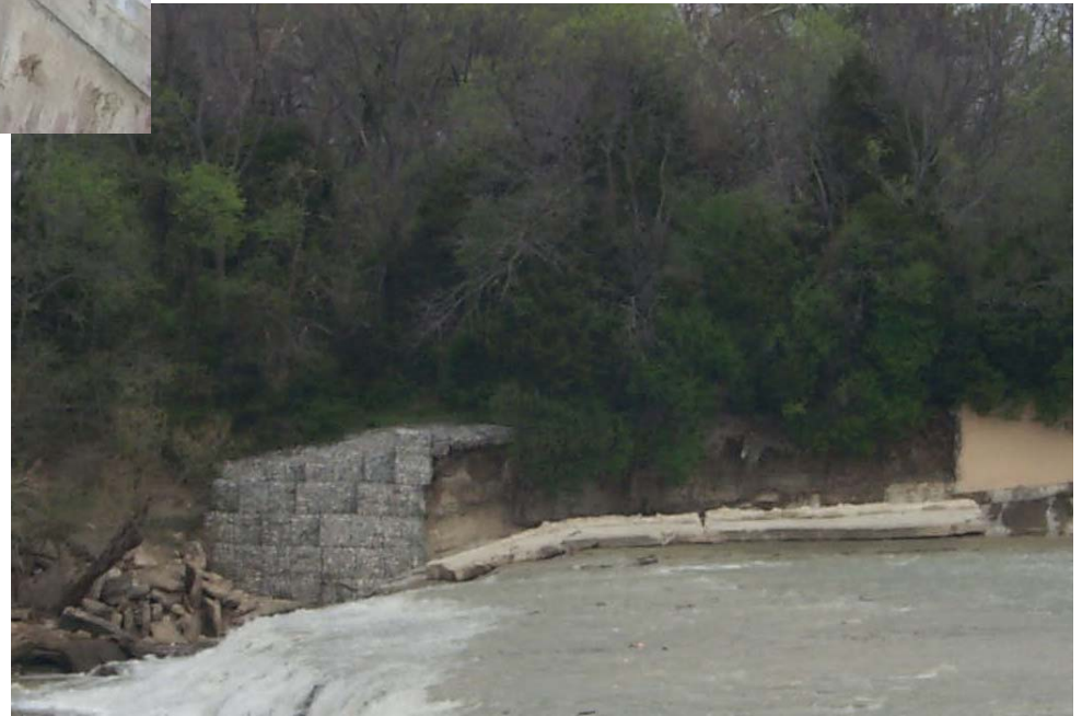
Retaining wall shear failure on north side of the Spillway
