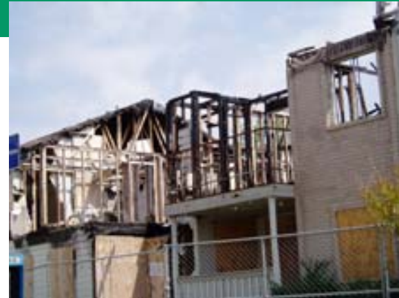
Units with fire damage
