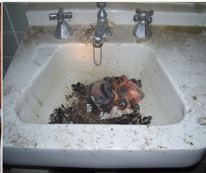
Pigeon infestation due to missing windows.
