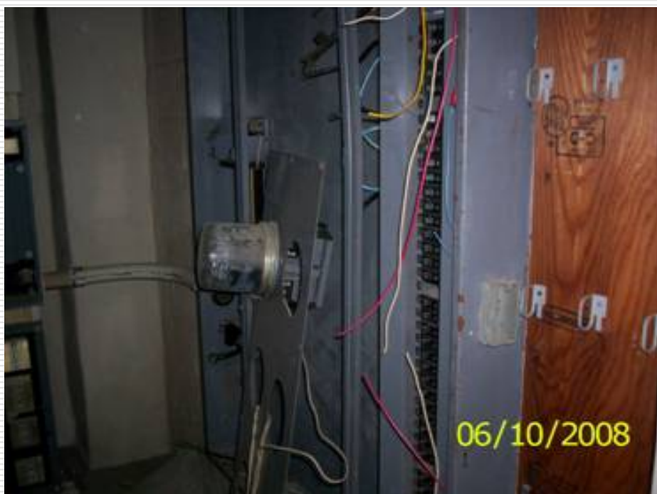
Exposed electrical. Copper stolen out of this unit.
