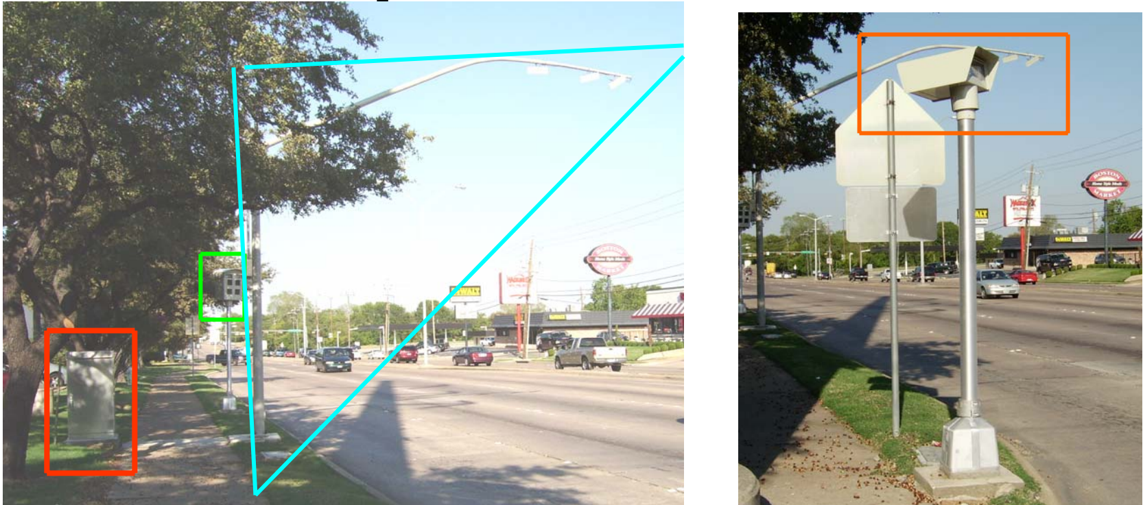
ACS camera system at Centerville and Northwest in Garland Texas. Cabinet , Camera , Speed detectors and Camera flasher .
