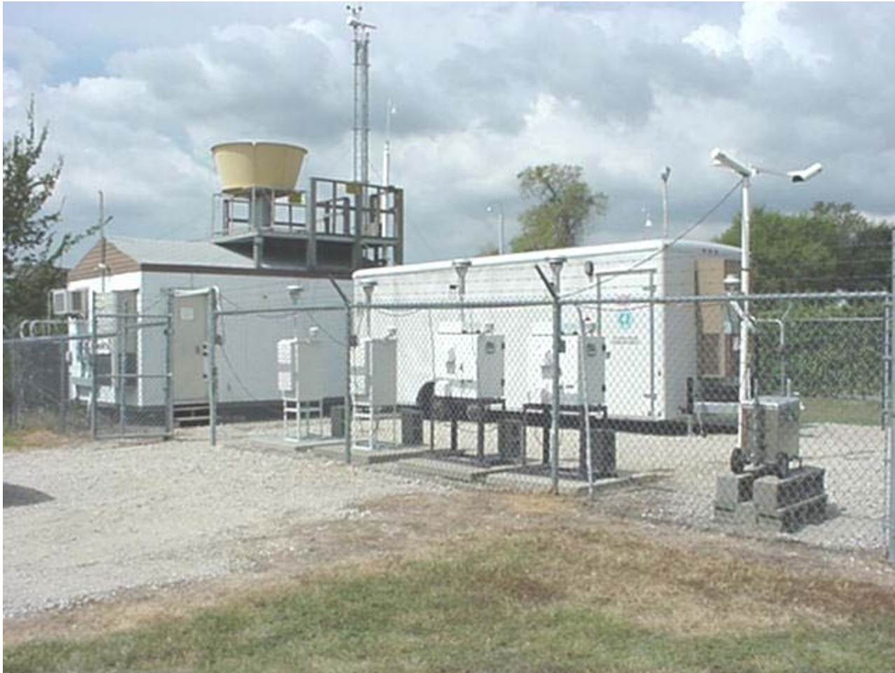
Typical Air Monitoring Station
