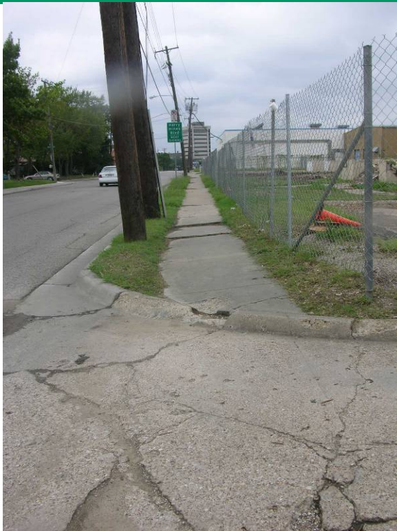
Narrow, cracked sidewalk on Butler Street
