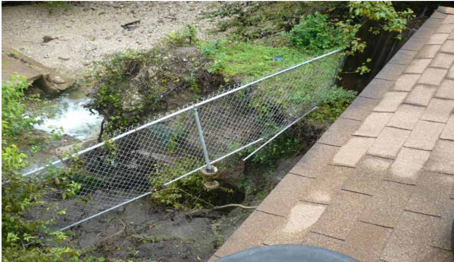
Creek erosion near top of bank and near home
