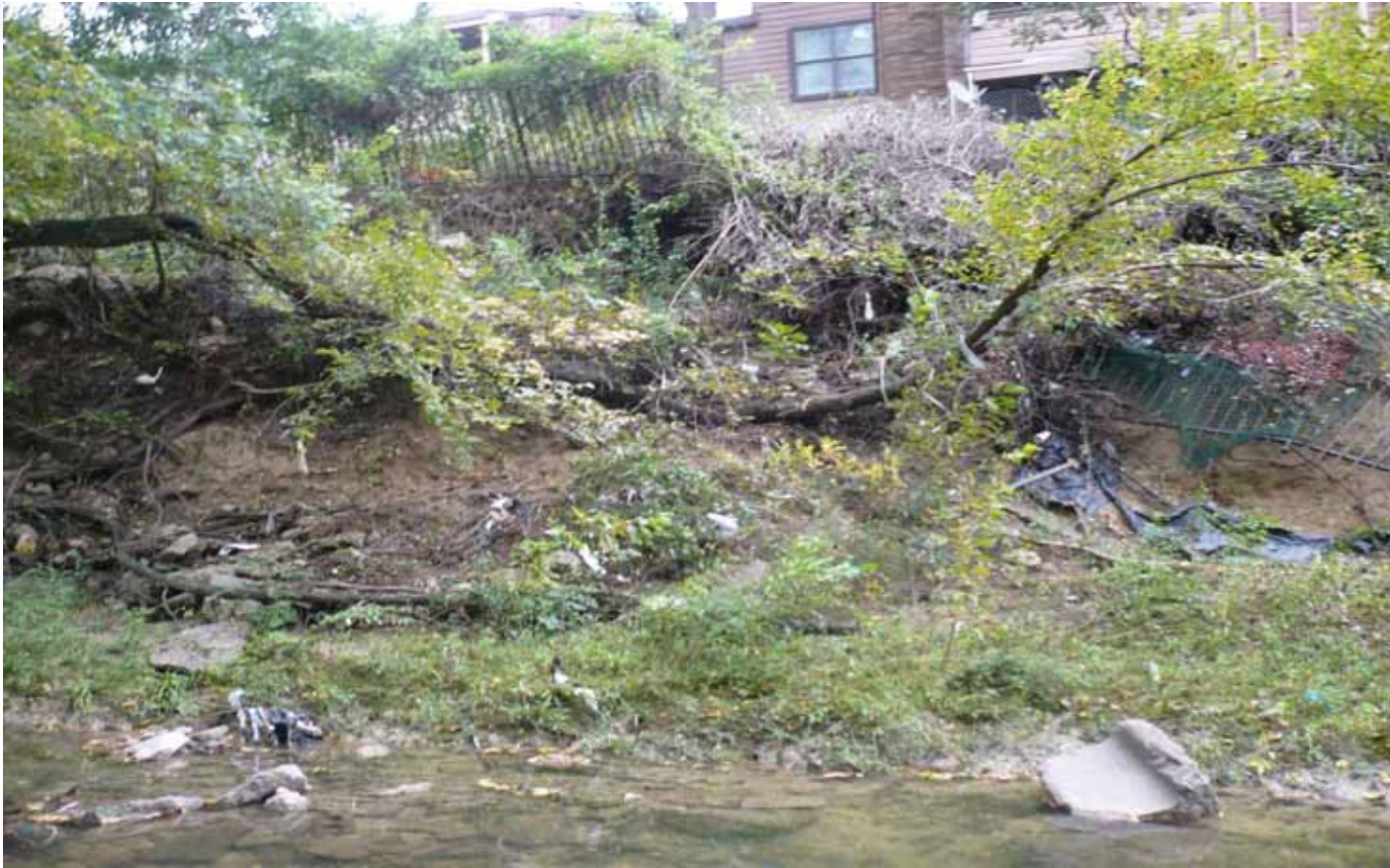
Slope failure near top of bank
