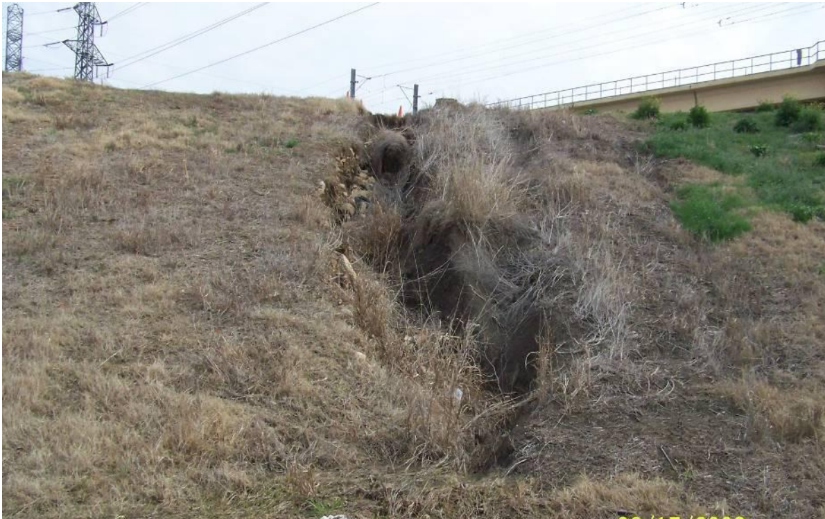
Sump Erosion Corrected – Able Sump
