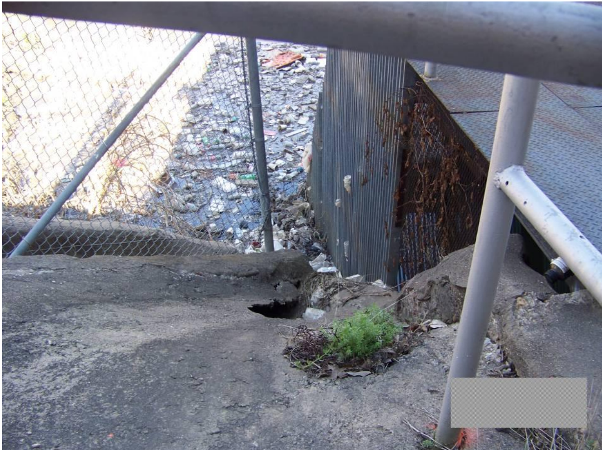
Damaged Concrete Flume – Able Station
